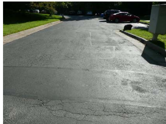
Yorktown Village Pass; note prior patch and extensive surface cracking
