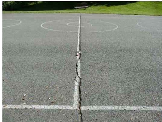
Basketball court; crack along mid-court
