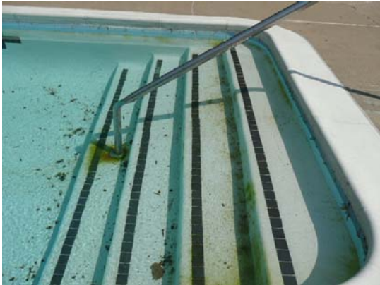
Main pool surface; note rust at rail
