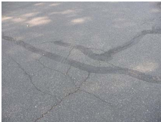
Yorktown Village Pass; note filled cracks and new cracks
