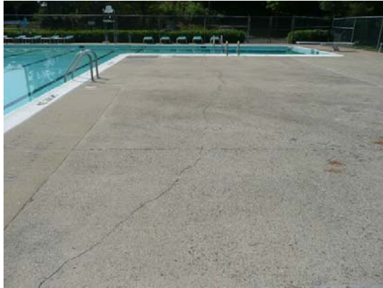
Cracked pool deck; typical condition
