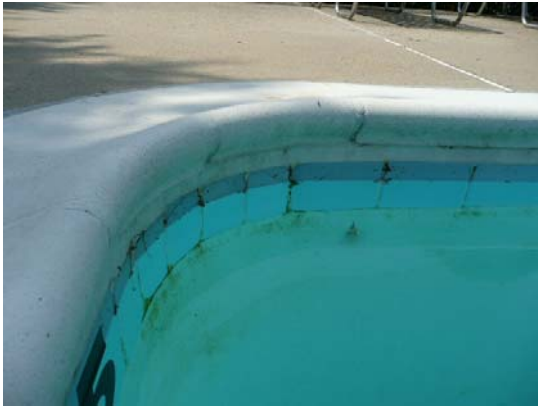
Main pool tile and coping; note green growth
