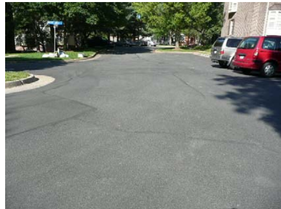
Butterfield Lane/Mount Airey Lane; note prior patches
