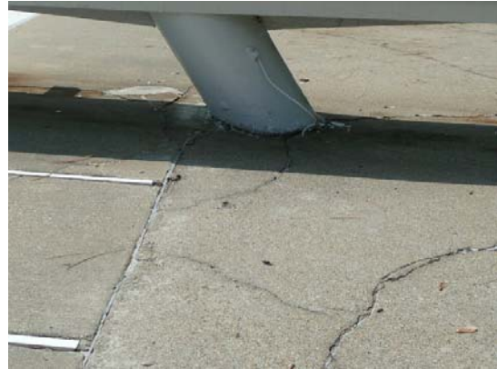
Cracked and settled concrete at diving board stand
