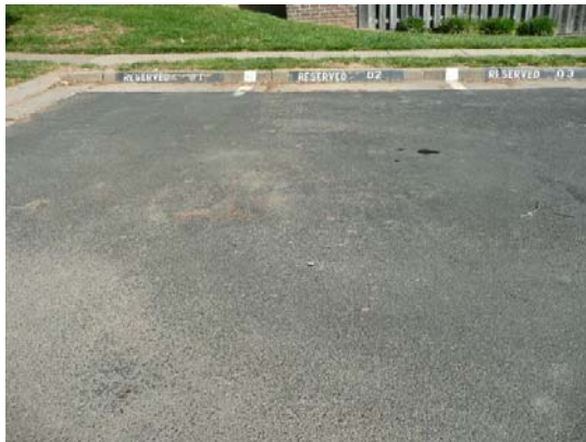
Butterfield Lane/Mount Airey Lane; note extensive surface cracking at parking spaces
