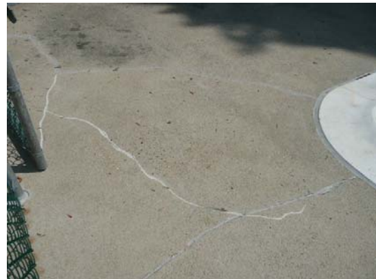
Cracked pool deck; typical condition
