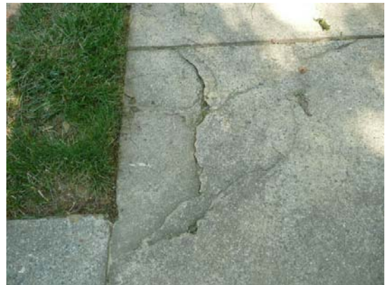
Cracked and settled section; typical
