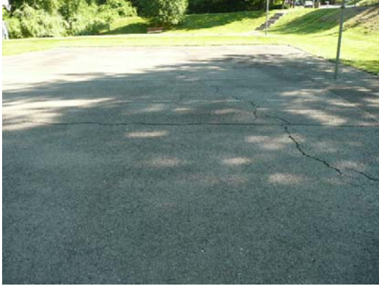
Volleyball court; extensive surface cracking
