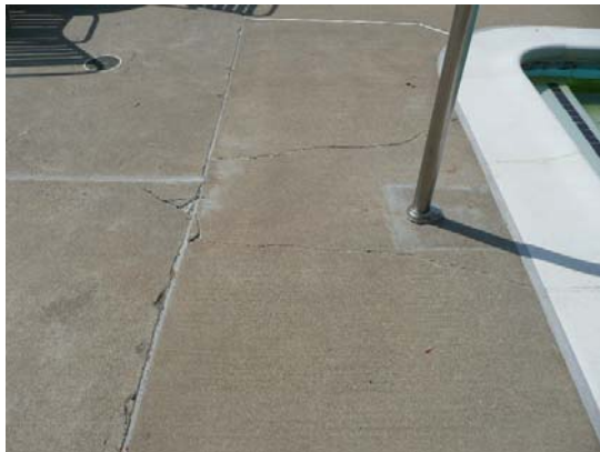
Cracked pool deck; typical condition
