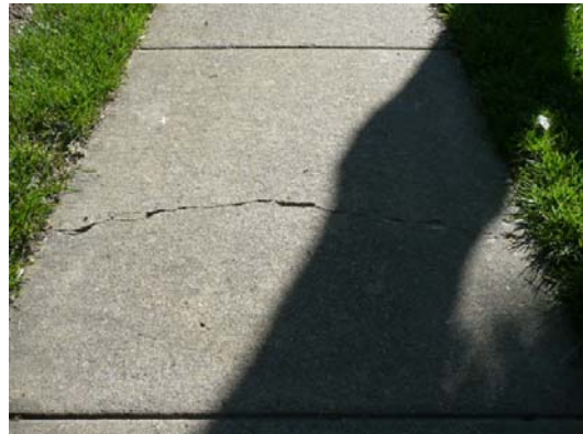
Cracked sidewalk section; typical
