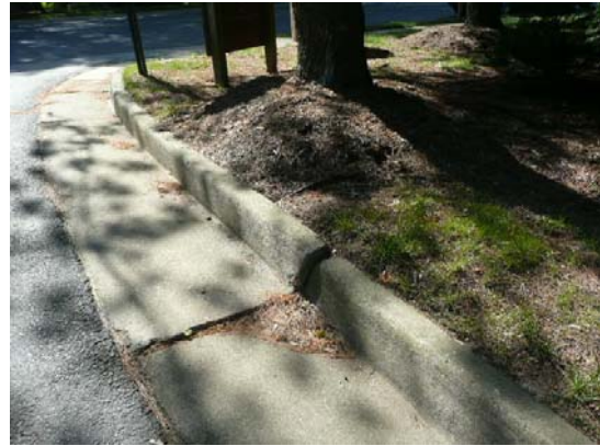
Heaved curb section; not typical
