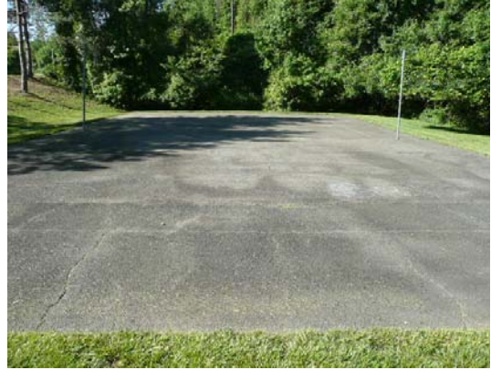
Volleyball court; extensive surface cracking and depressions
