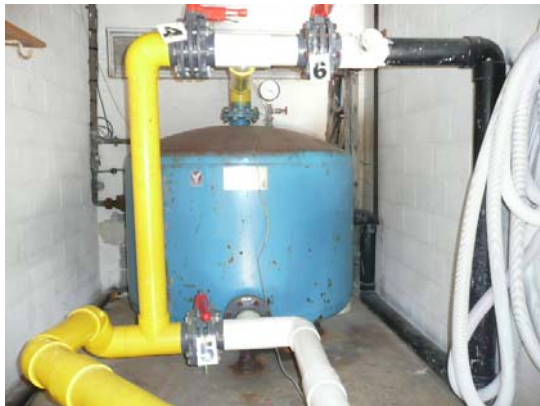
Main pool filter system; note corrosion on tank
