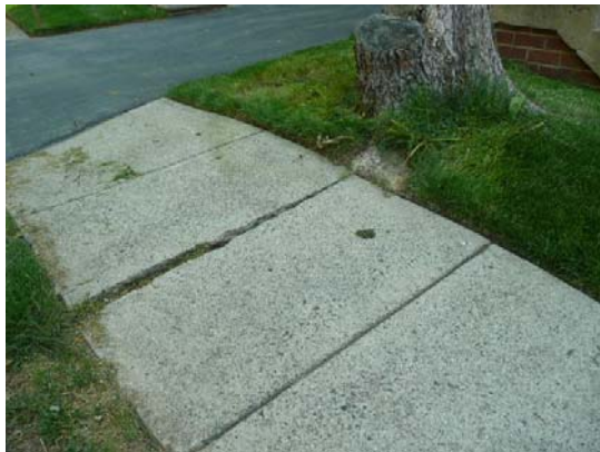
Heaved and cracked sidewalk section; typical
