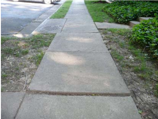
Heaved sidewalk section; typical
