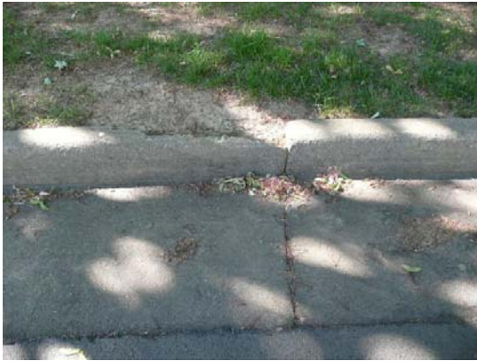
Chipped curb section; not typical
