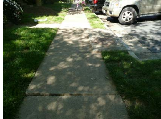
Heaved sidewalk section; typical
